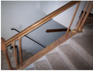
Interior Missing Railing
