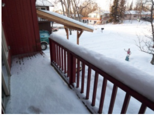
Exterior Missing Railing
